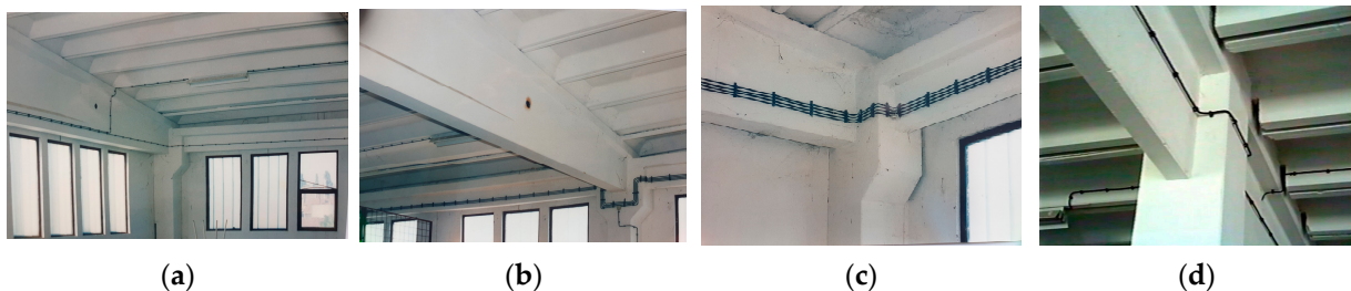
Figure 4. Connections of the existing industrial hall “Elektrotehna” in Nis, Serbia: (a) corner column—main roof girder; (b) mid column—main roof girder; (c) corner column—floor girder; (d) interior column—floor girder above the ground floor.
